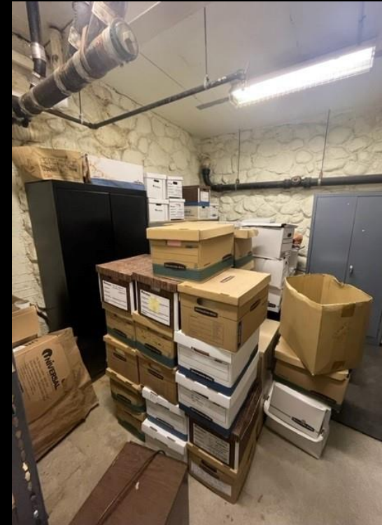
Fire District records retention area also has water infiltration
