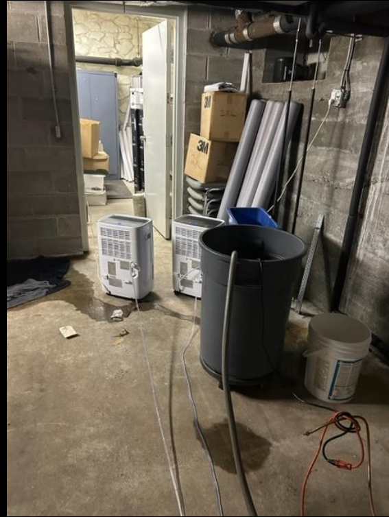
Dehumidifiers, buckets, and sump pumps to address water issues
