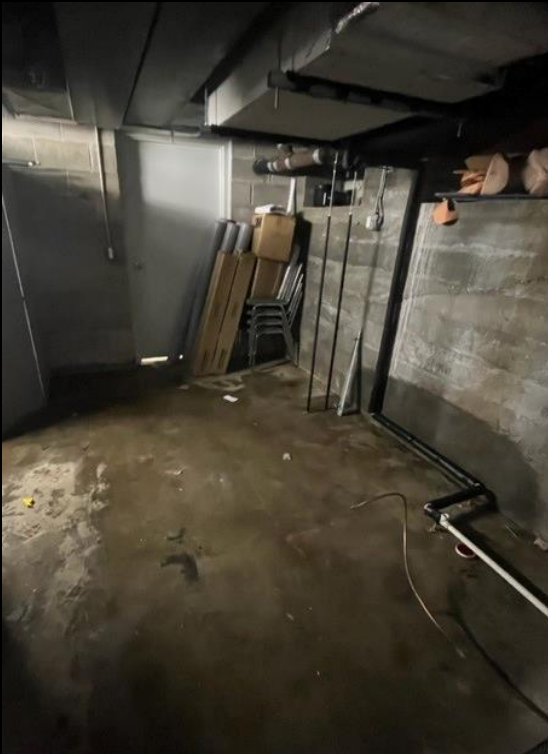
Storage room flooding caused by HVAC system
